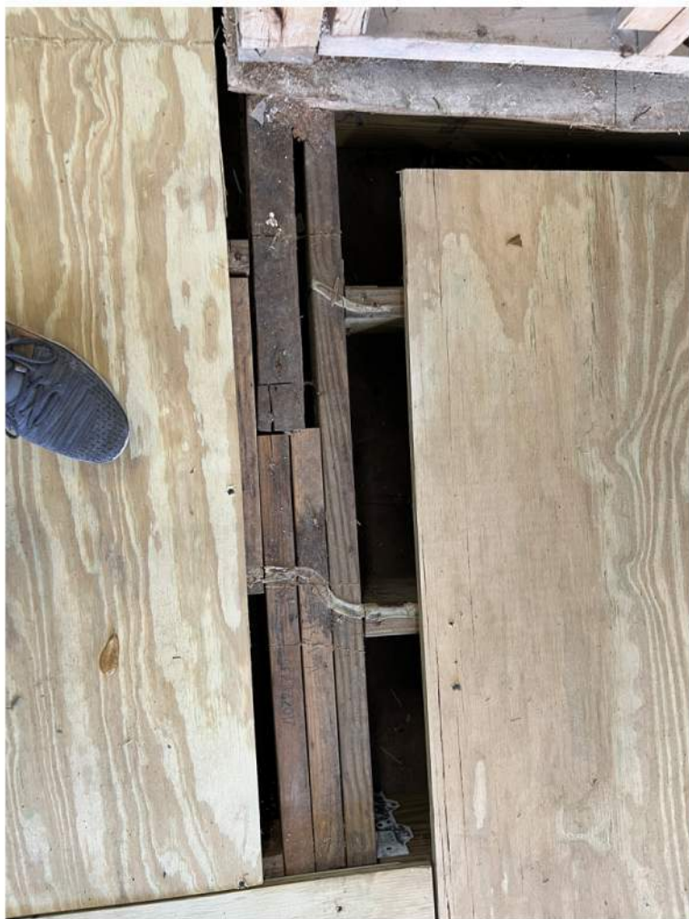
Improperly Lapped Floor Joists
