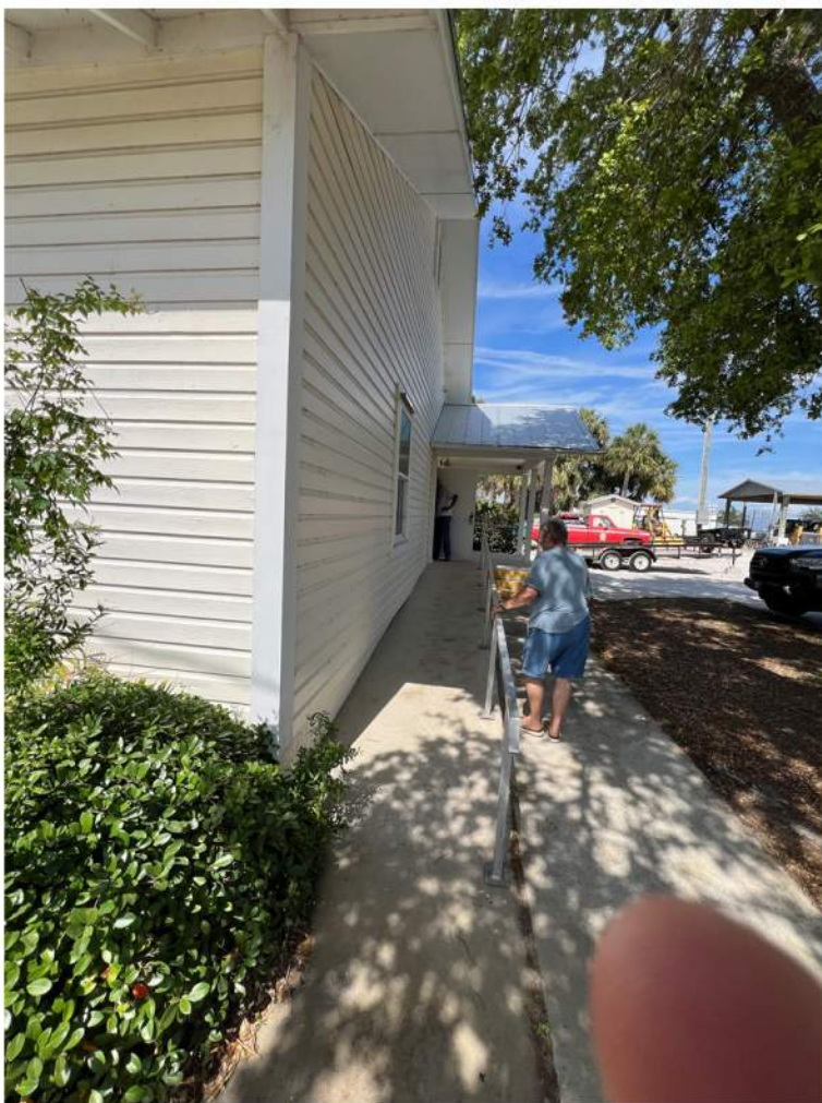
Ramp - Not ADA Compliant
