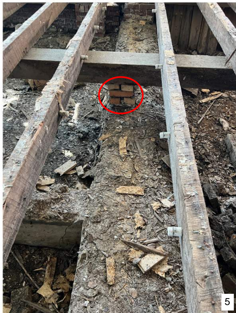
Floor Joists Unattached to Brick on Original Concrete Foundations
