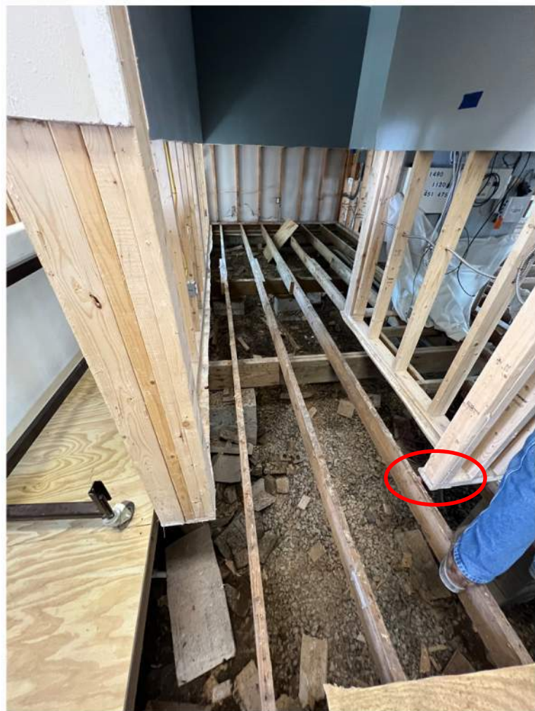
Floor Joists not Anchored to Foundations
