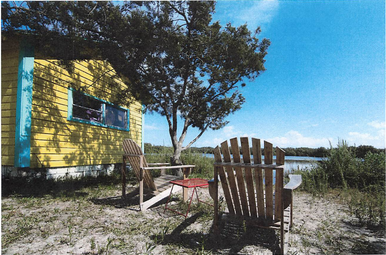
Current sea level often swamps this cottage at higher tides, frequent salt water inundations have weakened the foundation to near dust.
